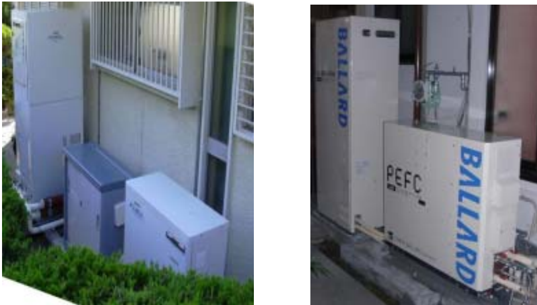
Fig.11 PEFC cogeneration systems at real customers' houses
