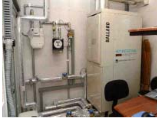
The wooden hut also houses a 200-liter hot water tank and a computer for collecting data.
