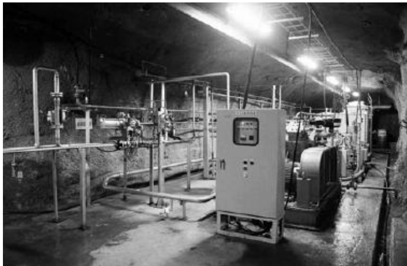
Photo 4: Pump and Compressor for pressurization of test cavern
