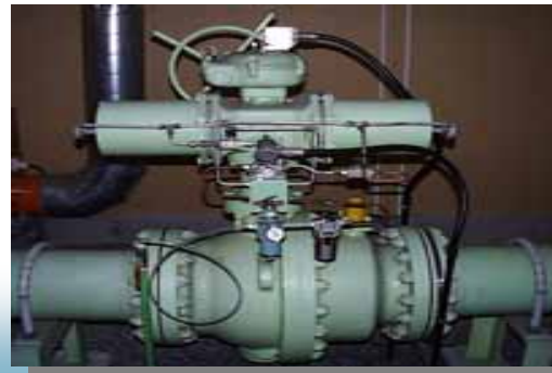
Remote shutoff valve
