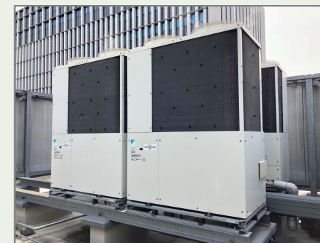
GHP 168kW (56kW×3台)
